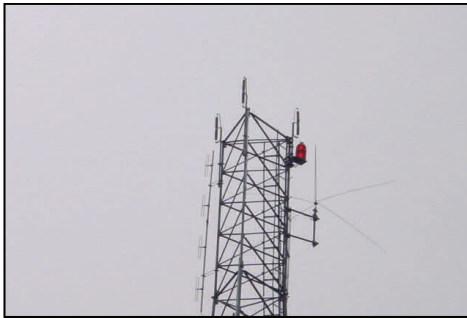
ALS-1000 air terminals on communication tower
