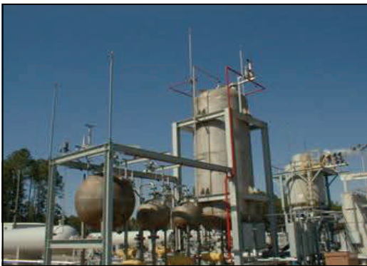
ALS-100 air terminals NASA fuel Facility
