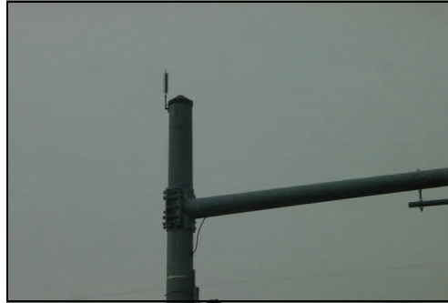
ALS-100 Air Terminal on NJ Expressway sign
