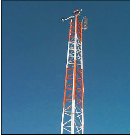
ALS-1000 Air Terminal on weather tower
